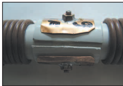
Condensatori in opera
